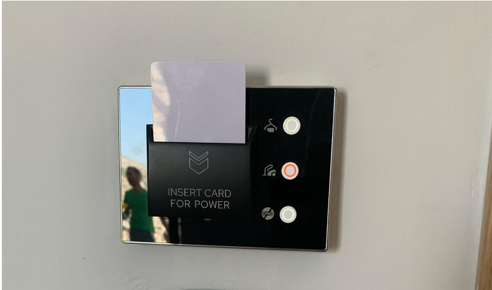
IO Switchcard has 3 mechanical keys installed inside the room
